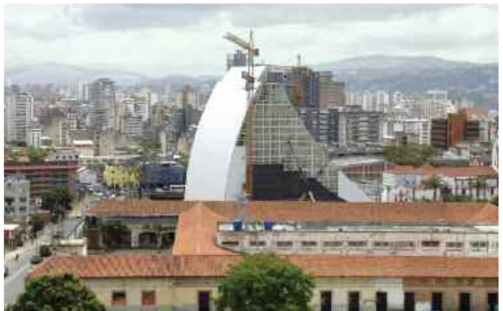
Figure 7 The new Mausoleo del Libertador (Liberator's Mausoleum) under construction, 2012. PHOTO: Gabriel Méndez.
